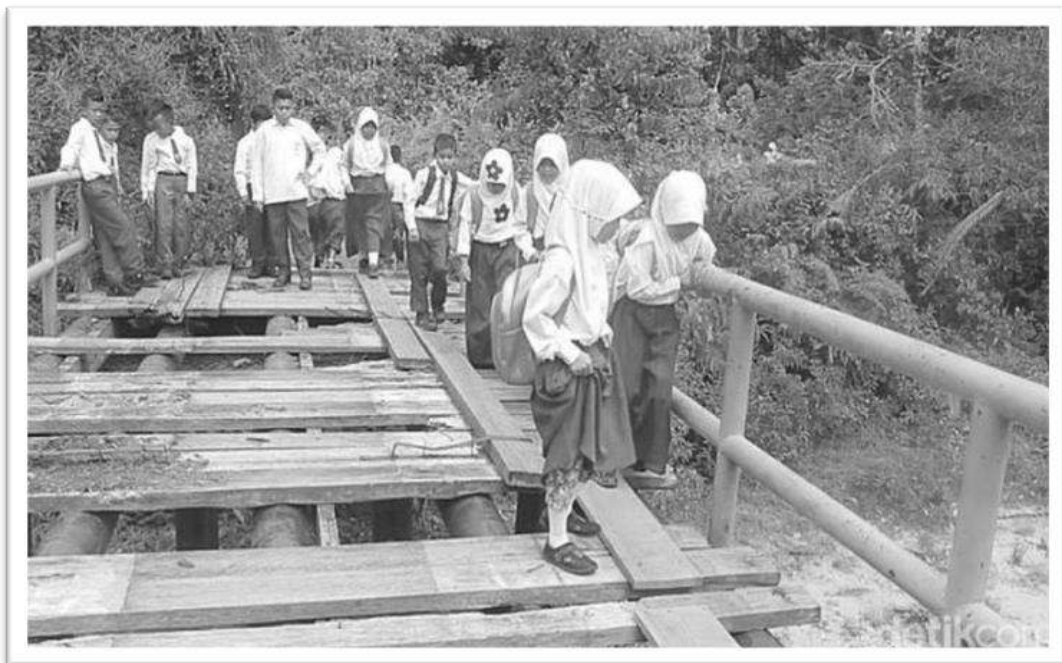
Figure 1.1. Kampar Regency, Riau. For the sake of schooling, elementary school students in Riau dared to cross the broken bridge.
