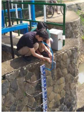
Fig. 13. Process installation sensor JSN-SR04.
